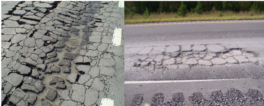
Figure 2.5.5: Fatigued sections N1 (left photo) and N2 (right photo).
